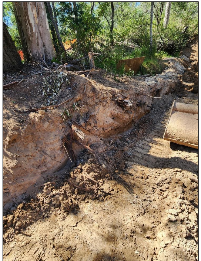
PHOTO 2 – Roots severed during excavation works within the SRZ.
