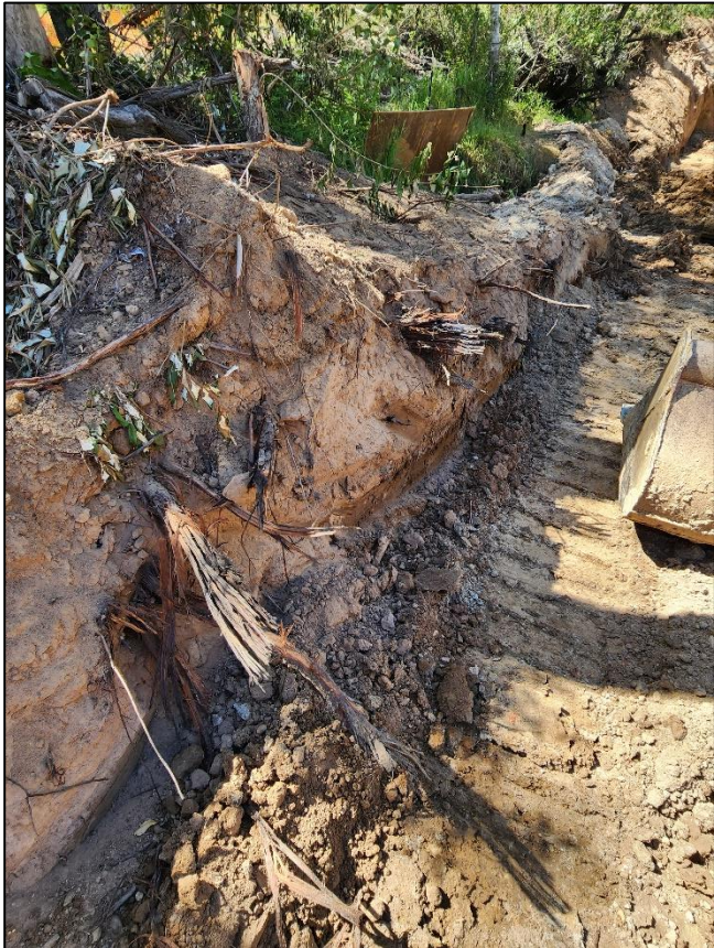
PHOTO 3 - Roots severed during excavation works within the SRZ.
